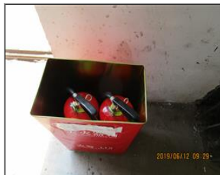
Photo of fire safety equipment Fire extinguishers.JPG
