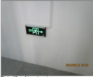
Photo of fire safety equipment Evacuation sign.JPG
