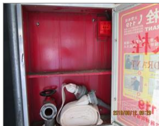
Photo of fire safety equipment Fire hydrant.JPG
